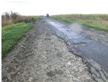
Figure 2.5: Section of asphalt road with broken surface and holes
